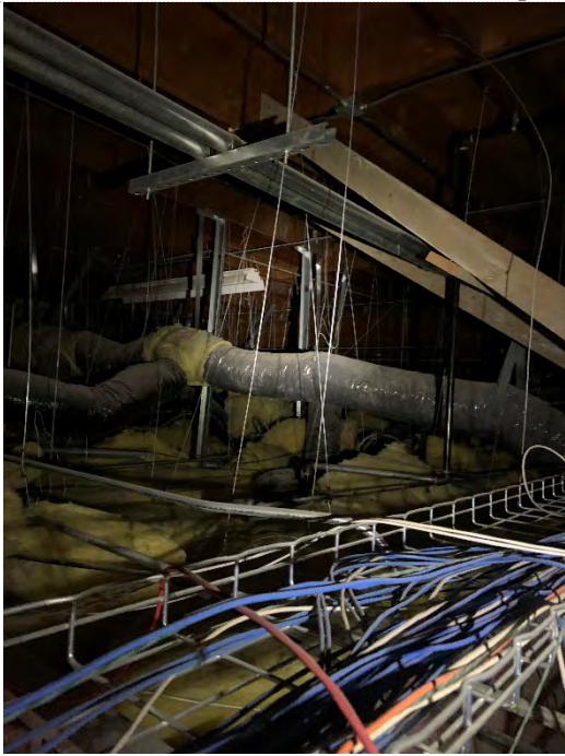
HVAC Ducting Overview – Fiberglass
